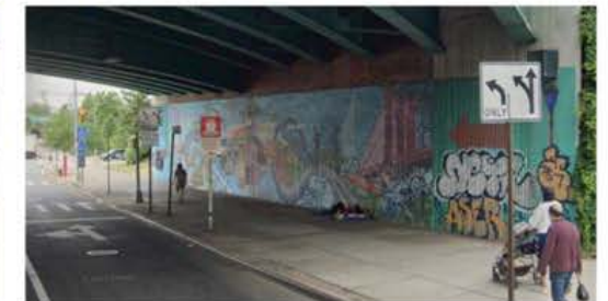
2 - Dark, Poorly-Lit Condition Below BQE Bridge
